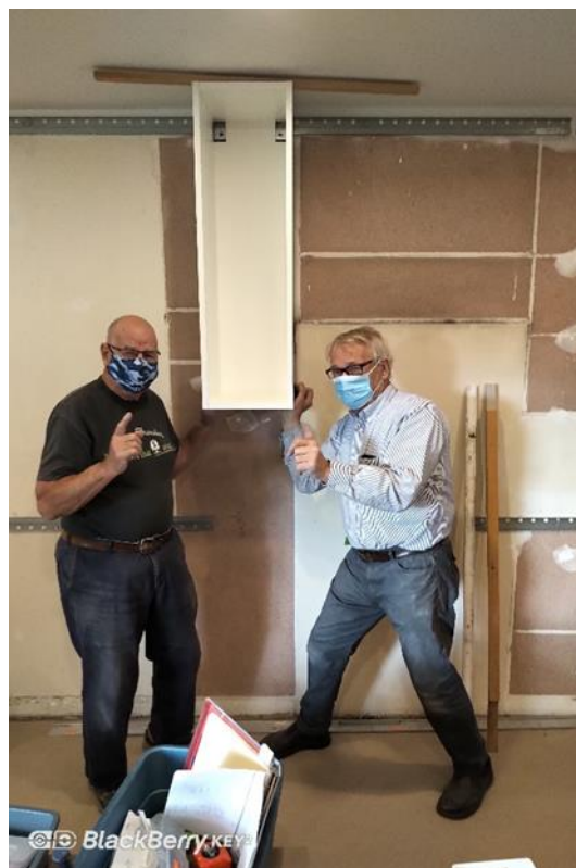
Art Schelter and Martin Juergensen having fun while they install cabinets in the kitchen of 235 Dawson Street.
