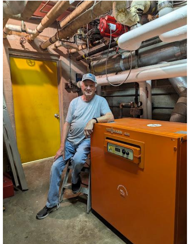
Ross Schlegel with original boilers which he installed 30 years ago.
